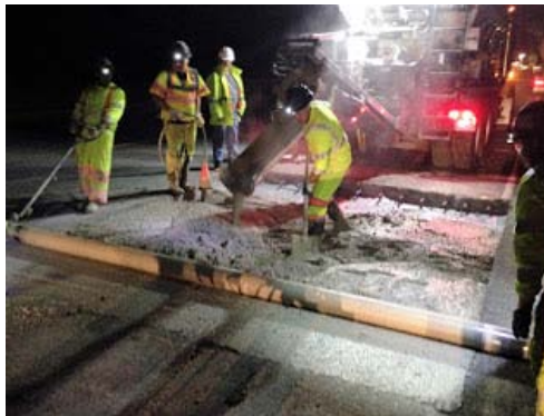
Replacing concrete panels on I-5 near Woodland is tough work, and keeping them safe is our top priority.
