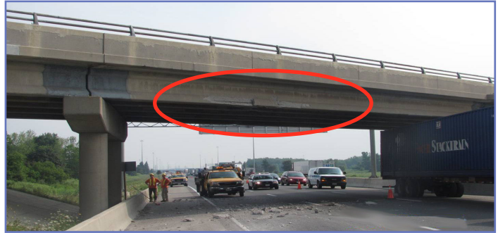
Damage to the Dingman Drive Bridge, looking eastward.
