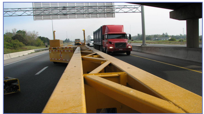
Mobile Traffic Barrier in use under the Dingman Drive Bridge.
