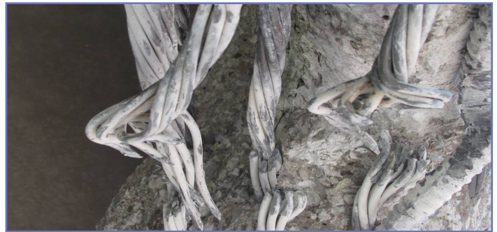
Collision-damaged strands on one of the bridge girders.
